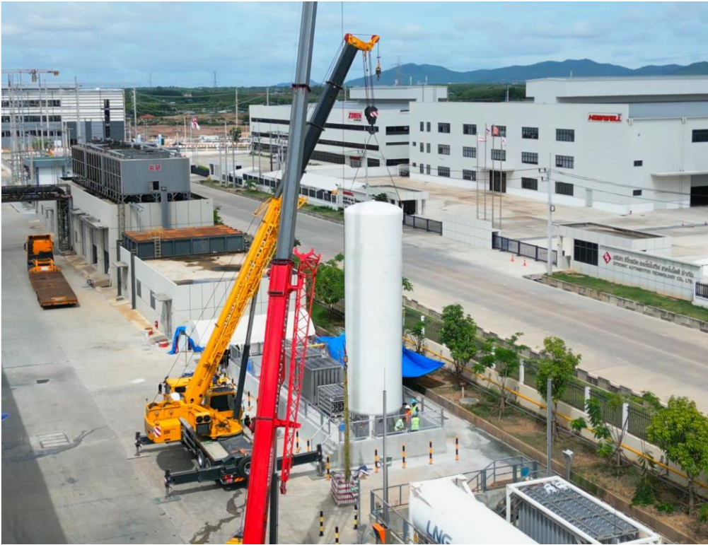
LNG Storage and Regasification Station
